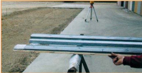
1. While the rails are still in a bundle, mark with a pen the position (see nr2) where the holders have to be fixed.
