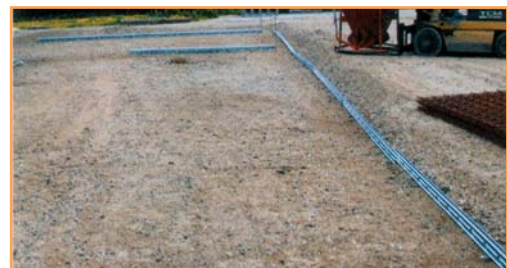
4. Lay the rails along the string, ensuring that the folded top is to the side that is to be concreted last.
